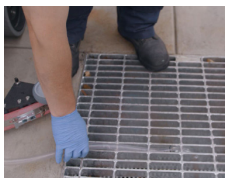
STEP 7 Empty solution tank
