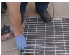
STEP 7 Empty solution tank
